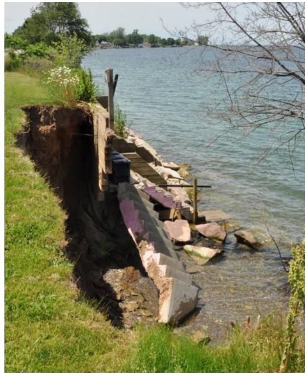
Example shoreline erosion conditions
